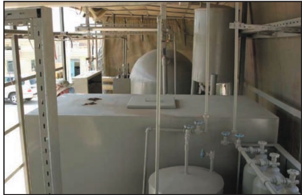
Interior view of fermentor, media tank, water supply tanks, and gas cylinders connected by pipes.
