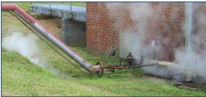
A failed-open steam trap can waste considerable steam.
