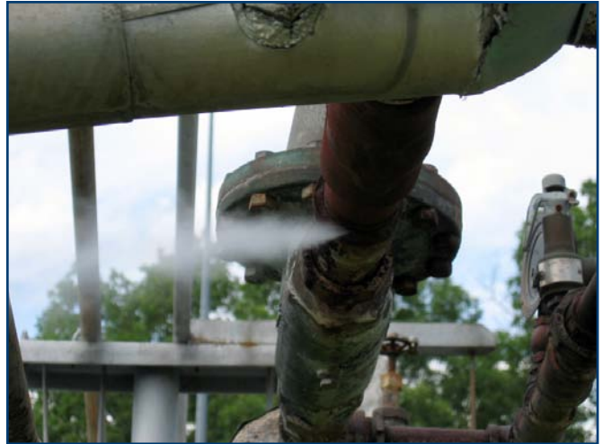
Steam leaks can be dangerous, as well as energy wasters. This uninsulated pressure-reducing station should also be insulated.
