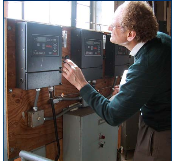
For larger systems, continuous and automatic trim-control systems should be considered.
