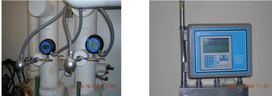
Figure 8.6. Chiller Water Metering at NIH. Photo on left shows water supply and return pressure sensors; photo on right is a chiller water meter energy/flow processor.
