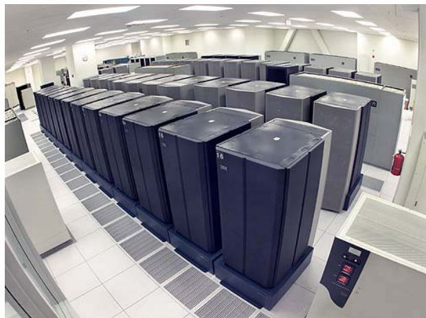
Figure 7.10. Typical Data Center
