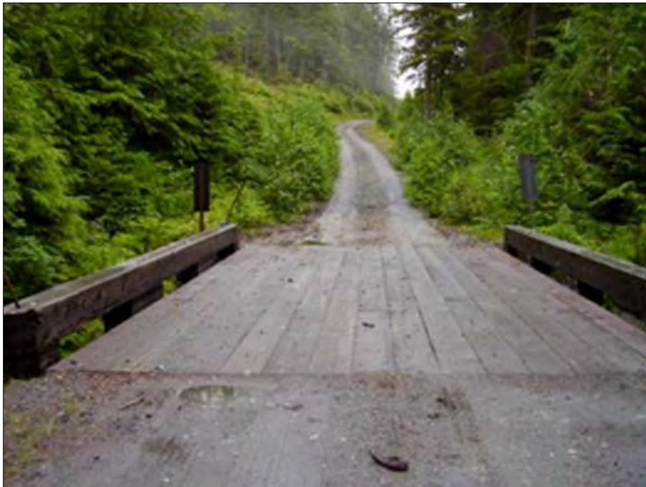
AFTER: Alaska (OIG Photo). This project included repairs to bridge decking, curbing, and guardrails.
