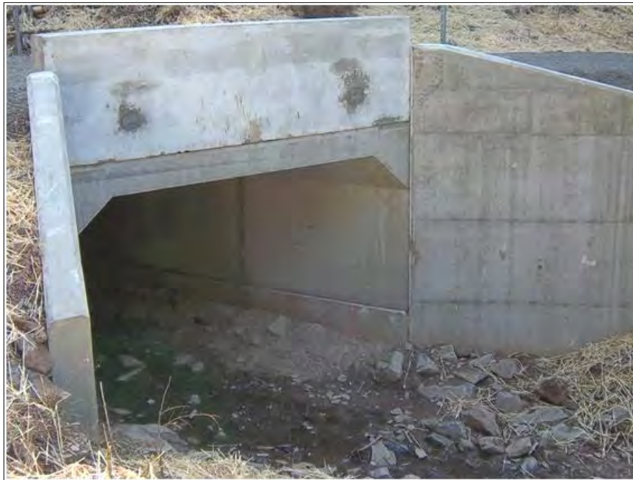
AFTER: Oregon (OIG Photo). The pipe culvert was replaced with an “aquatic organism passage” that allows not only fish, but other aquatic and terrestrial creatures to pass through (photo was taken in the fall). The straw on the banks helps to foster growth of the seed FS planted post-construction.
