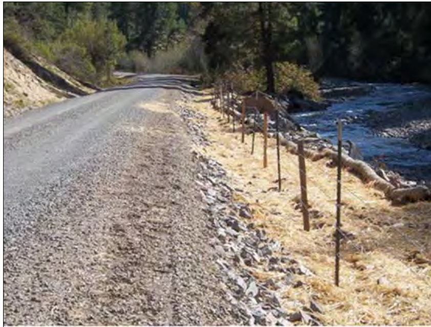
AFTER: Oregon (OIG Photo). Work involved shifting and raising the roadbed, placing rocks along the hillsides, rebuilding fences along the river side of the road, and replacing culverts and cattle guards. Afterwards, the hillsides were seeded and mulched.
