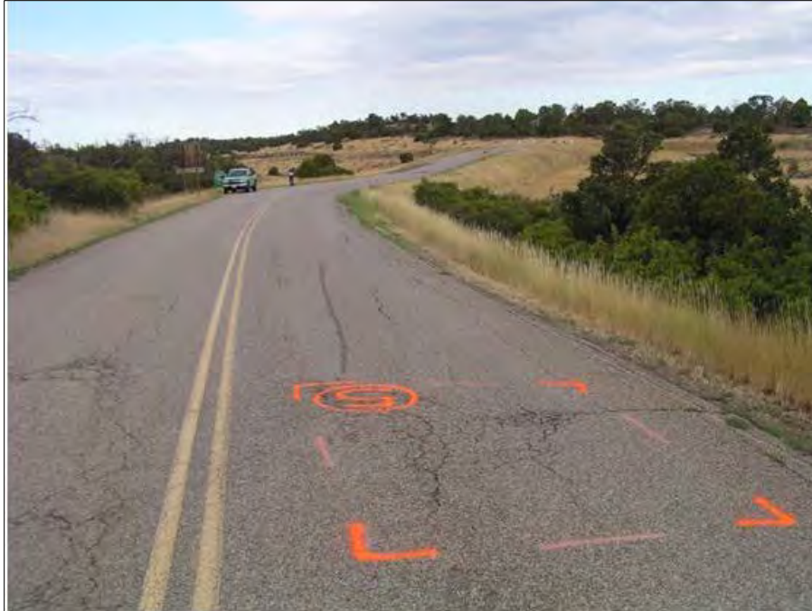
BEFORE: Colorado (FS Photo). FS Road 271 provides access to McPhee Marina. Over the past 25 years, the road slowly deteriorated.
