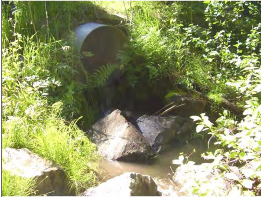
BEFORE: Oregon (FS Photo). This 48-inch pipe culvert on a service road off of FS Road 7700 did not allow for fish passage (photo was taken in the spring).
