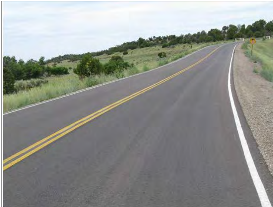
AFTER: Colorado (OIG Photo). This project involved repaving the road since a chip or crack sealing would not have been effective.
