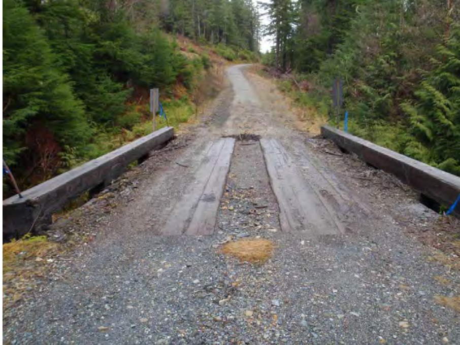
BEFORE: Alaska (FS Photo). This bridge was missing several running planks of bridge decking.
