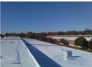
Figure 5: Energy saving cool roofs.
