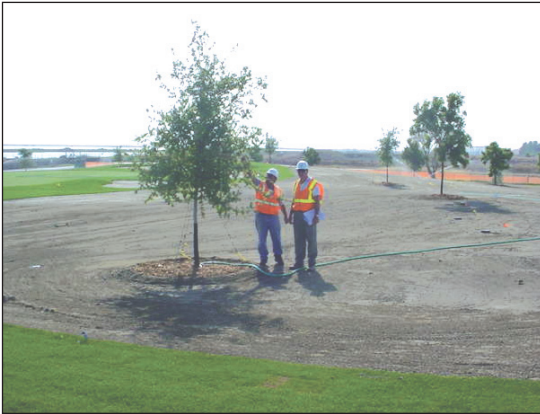
The Site 22 Golf Course Landfill is covered with a biotic barrier and restored. Rodent-proof casings protect trees that are aesthetically pleasing to the public and enticing to local birds of prey. The new trees are monitored and cared for regularly.
