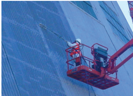
Contractors employed a number of innovative methods to seal Hangar 1's decaying surface quickly and safely.
