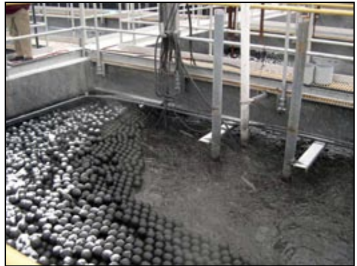
▲ Thermal balls are used in the Bioplant to retain heat in the winter, optimizing biological activity and digestion of waste solids.
