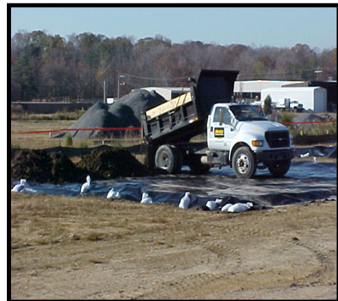
Stockpiling of soil on impermeable plastic liners during the OU 4 Removal Action.
