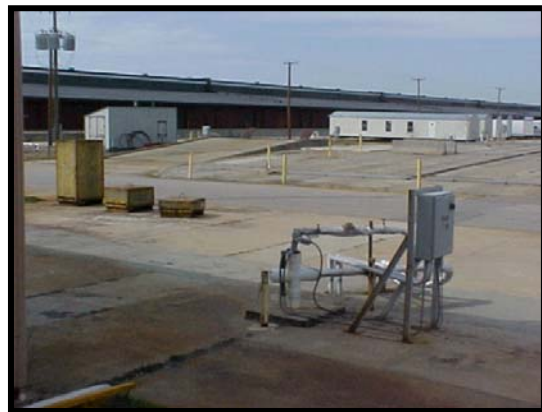
Dual-phase extraction well for OU 8 treatment system
