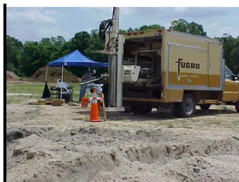
Direct Push Technology (DPT) sampling used to identify source material at OU 4.
