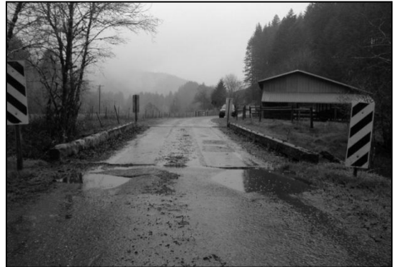
Bridge approach work is a typical ongoing maintenance need for western Oregon roadways. Ditch clearing needs and culvert replacements are also in constant demand.
