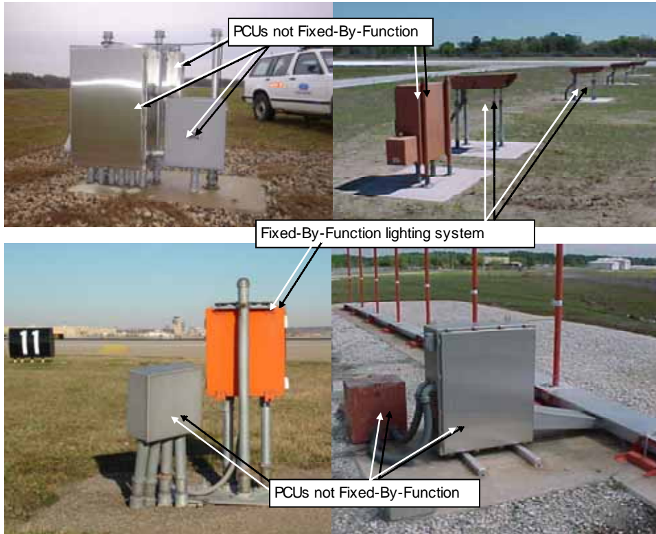
Power/control units (PCU) and junction boxes that are not fixed-by-function
