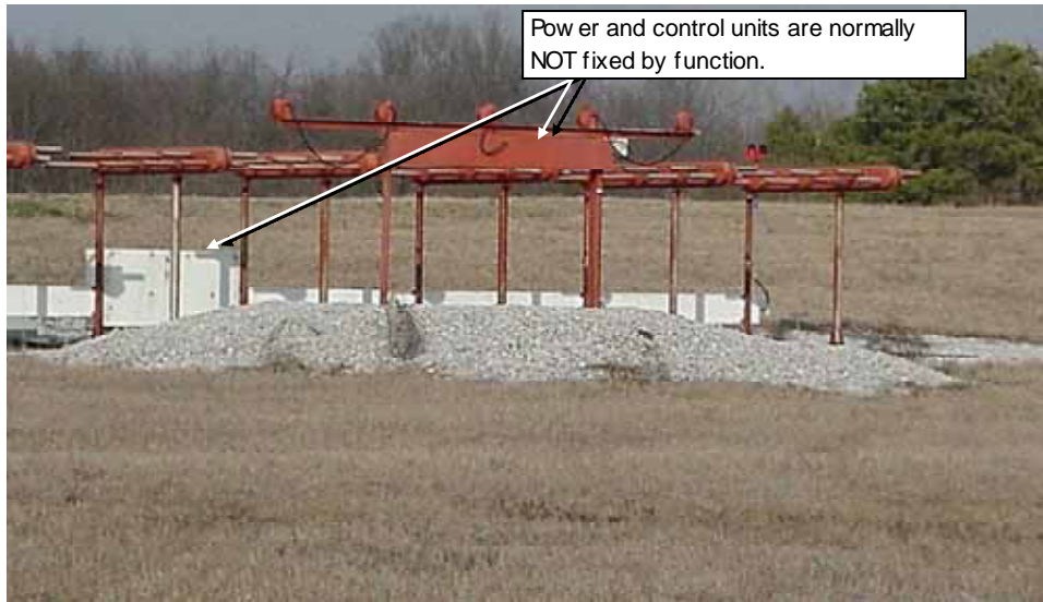
Excessive gravel fill creates a hazard
