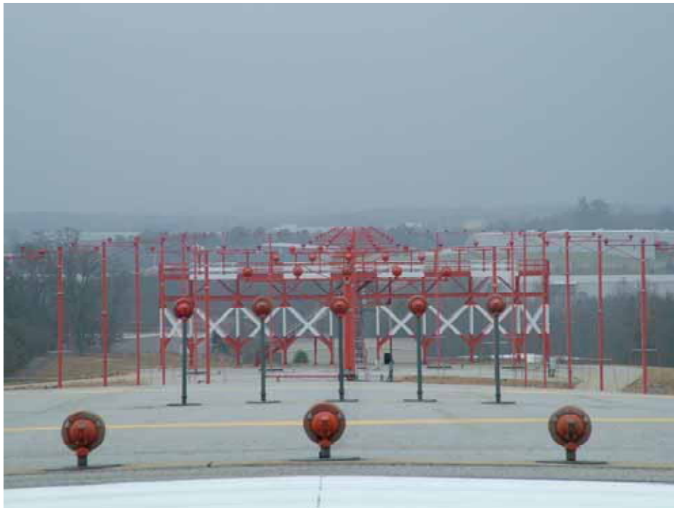
Standard ALS installation. Note electrical metallic tubing (EMT) with frangible couplings installed on light stations that are less than 6 feet high.
