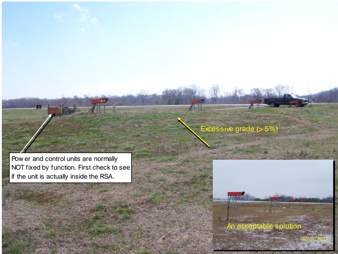
PAPI installation with excessive grade
