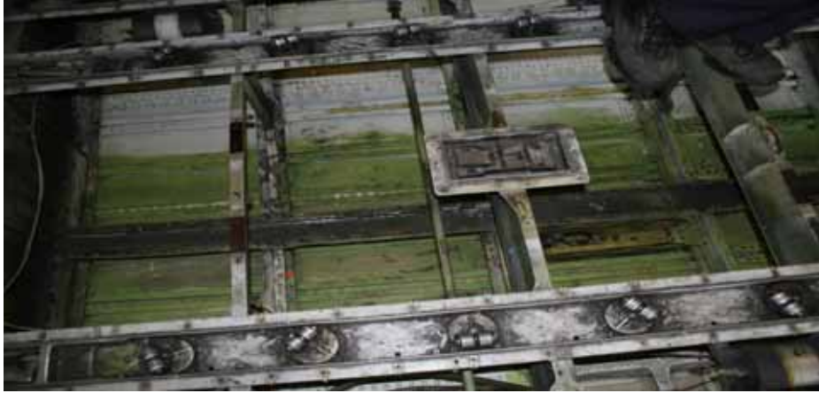
Figure 5-2. With the lower deck floor removed, the bilge bays can be more clearly seen. Water from firefighting will accumulate in the bilge.
