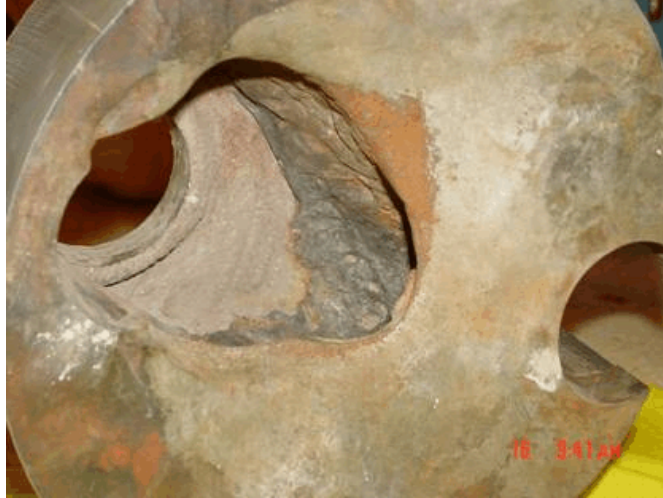
Figure 4. A photograph of the 18-inch diameter section of the discarded Davis-Besse head, containing the corrosion cavity created by leakage from the included nozzle (#3). The hole at the right is from nozzle #11.
