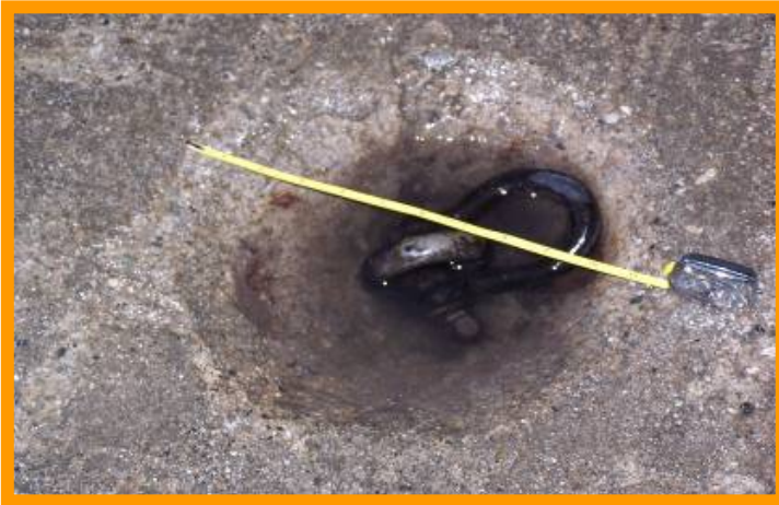
A hole, located in a holding pen floor with a metal staple and ring attached to the base of the hole that may cause an animal to fall or result in injury to feet.
