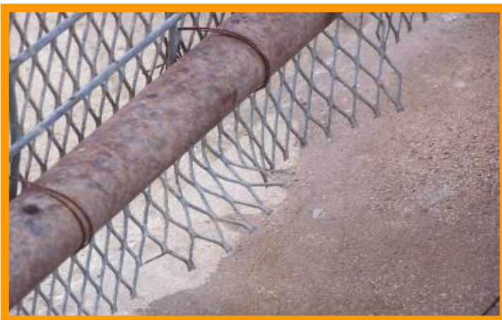
Bent fencing sufficient to allow injury to an animal's foot
