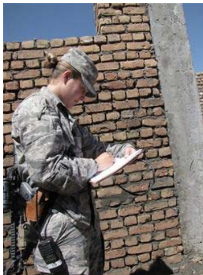
PANJSHIR, Afghanistan - A civil engineer with the provincial reconstruction team here, 1st Lt. Kate Miles takes notes on construction progress of a new government building Sept. 6, 2009. Lieutenant Miles and her team ensure contractors perform work according to code. She is a Rochester, N.Y., native and deployed from Luke Air Force Base, Ariz. (U.S. Air Force photo/Staff Sgt. J.G. Buzanowski)
