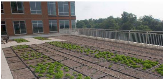
A “green,” stormwater-management roof on an EPA building in Arlington, Virginia (EPA photo).
