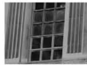
FIGURE 11 Exterior before (top two rows) and after (bottom two rows) views showing original windows and blast resistant replicas illustrating minor muntin-voiding needed to secure the thicker laminated glass of the new blast window. (Mariah McGaughey/GSA)
