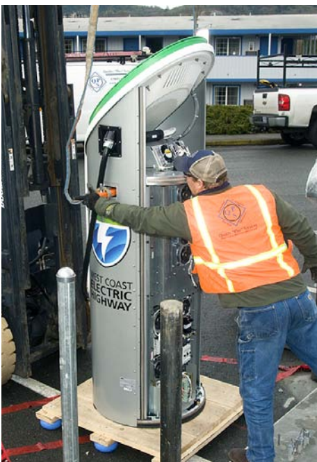
Workers install charging equipment in Grants Pass, Oregon. Photo from ODOT Photo and Video Services, NREL/PIX 20643
