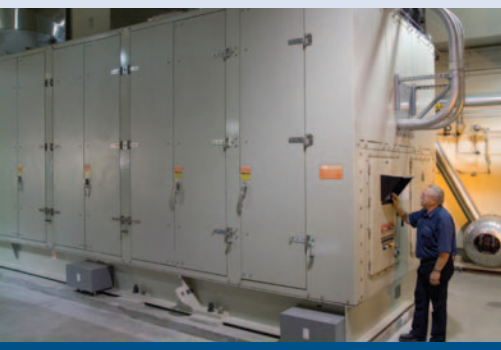
Veterans Administration Medical Center, San Diego, Photo Courtesy of Solar Turbines
