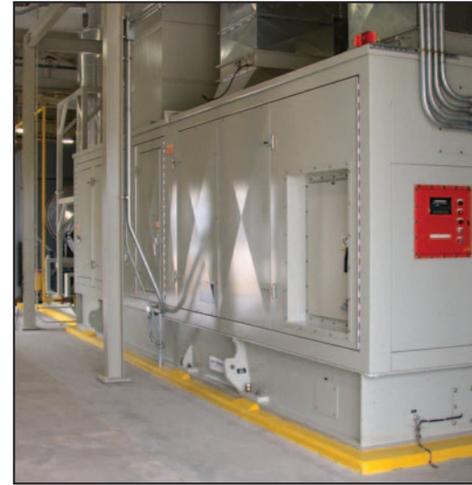
Domain Industrial Park, Courtesy of Solar Turbines
