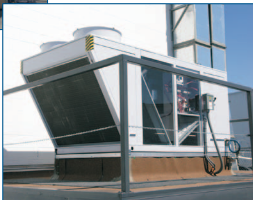
Gas Engine Heat Pump in Operation, Courtesy of Southwest Gas
