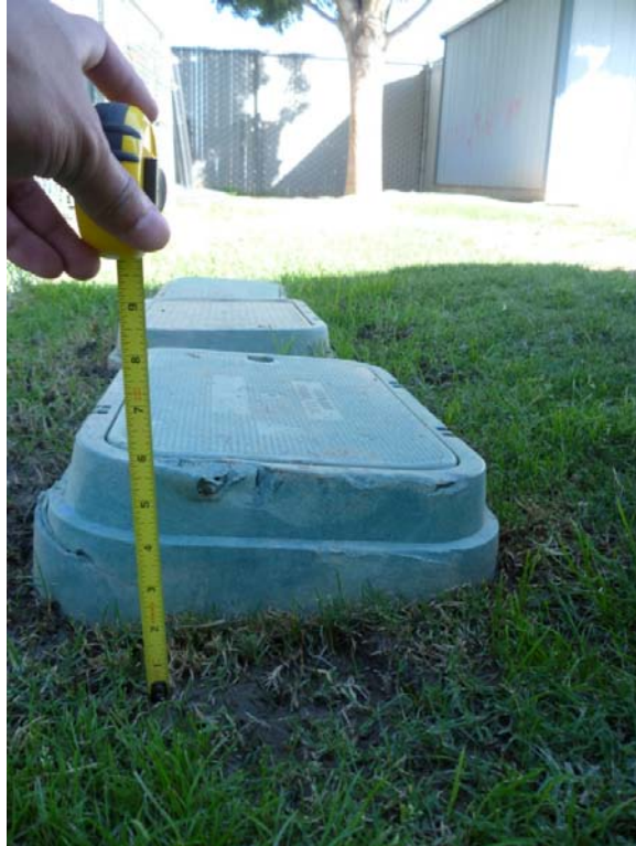
Photograph 3 – Taken at Preston Green on 10/14/10 showing irrigation control valve covers on the playground that presented a tripping hazard.
