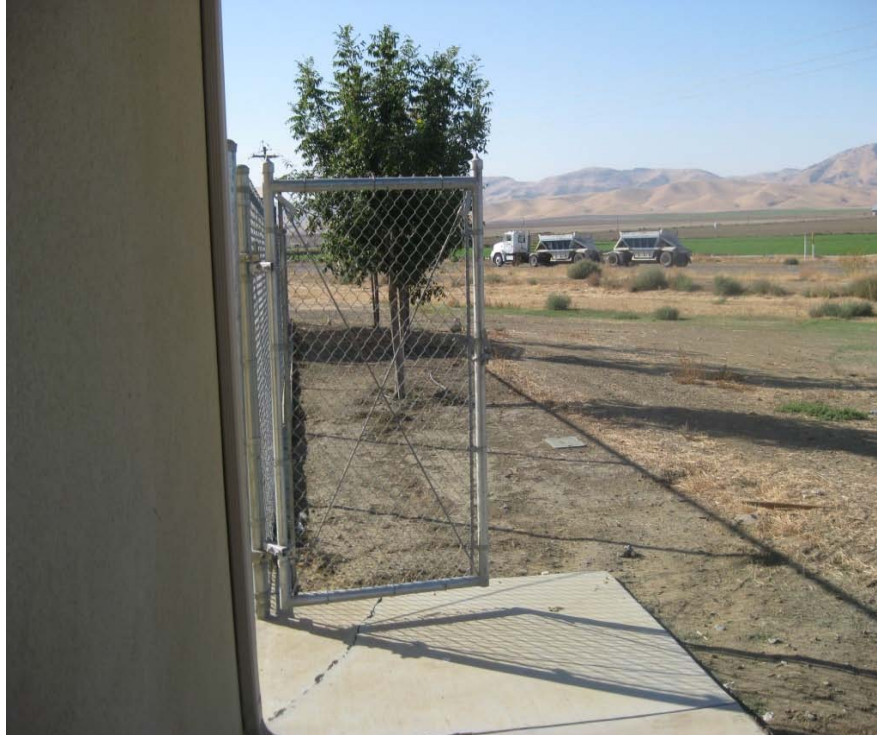
Photograph 7 – Taken at Oasis on 10/15/10 showing an unsecured gate on the playground that led to a busy road. The gate latch was within children’s reach.
