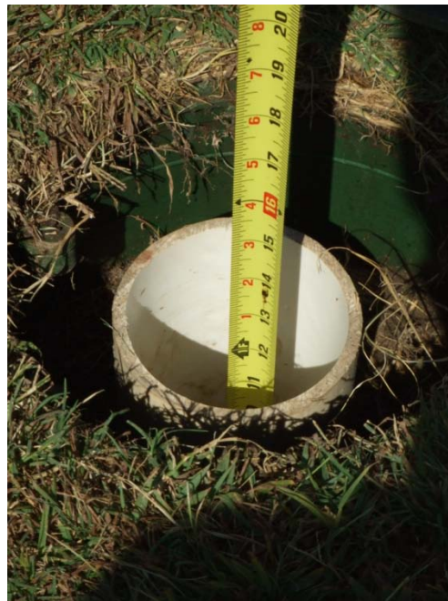
Photograph 6 – Taken at Generations on 10/14/10 showing a 15-inch-deep hole for an irrigation control valve with an unsecured cover (removed for photograph).
