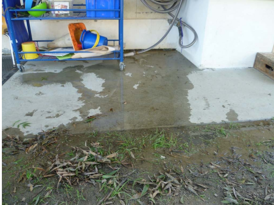
Photograph 5 – Taken at Preston Green on 10/14/10 showing muddy areas on the playground created by a leaking garden hose.
