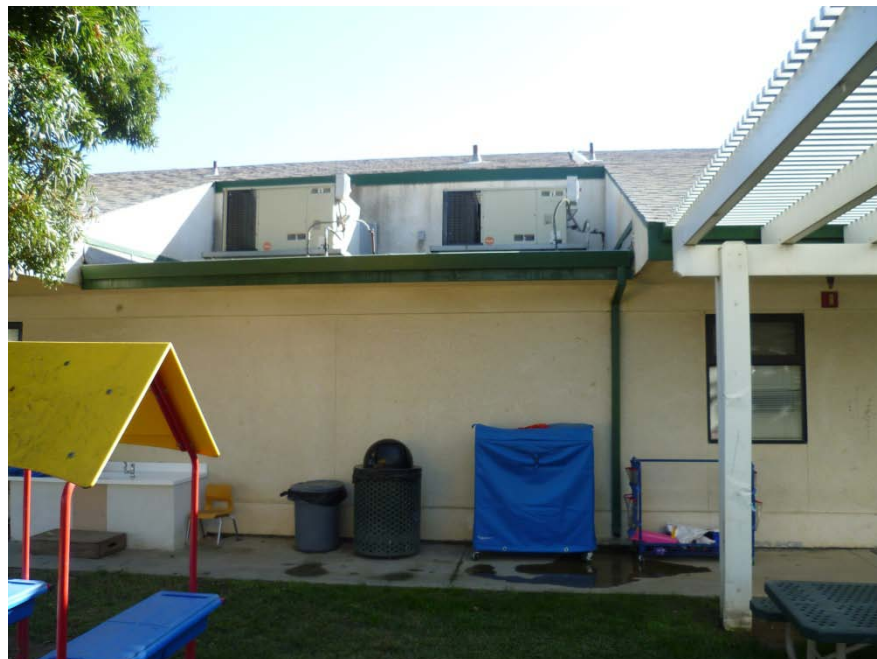
Photograph 4 – Taken at Preston Green on 10/14/10 showing a pool of water on the playground sidewalk created by drainage from an air conditioning unit on the roof.
