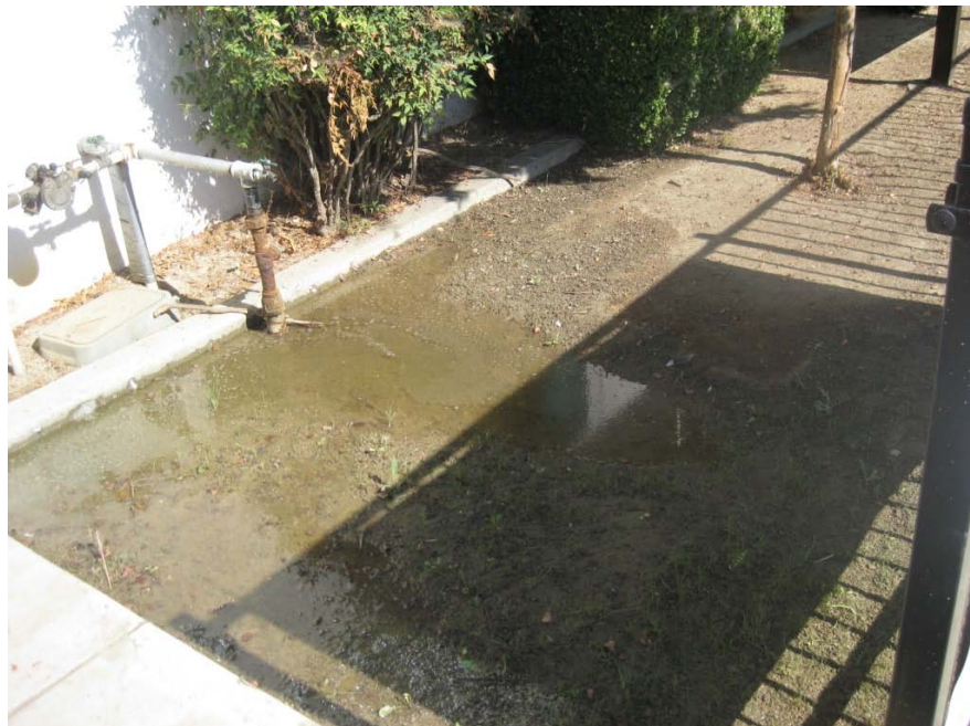
Photograph 8 – Taken at Avenal on 10/15/10 showing a large puddle of stagnant water adjacent to the sidewalk near the facility’s front entrance.
