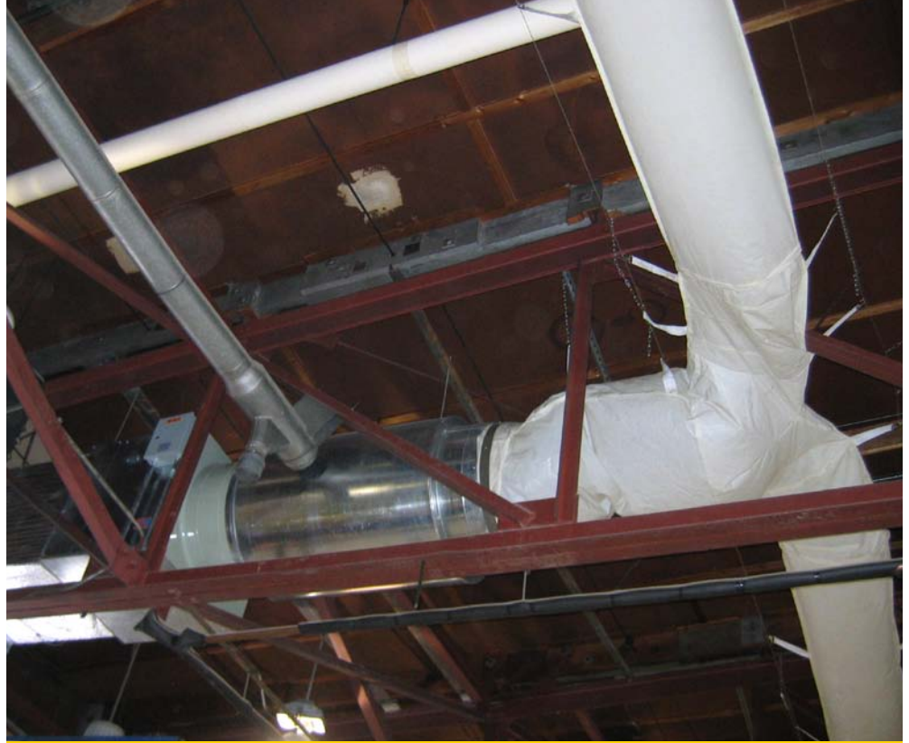
Fabric duct supplied with ventilation air. Photo by Ed Hancock, NREL/PIX 19364
