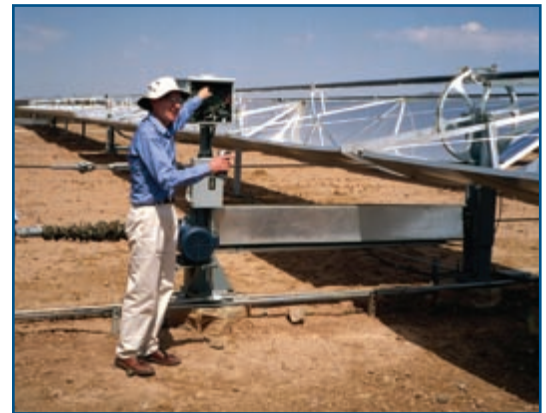
Parabolic trough concentrator modules at the Phoenix Federal Correctional Institution produce up to 50,000 gallons of hot water daily—enough hot water for kitchen, shower, laundry, and sanitation needs for 1,250 inmates and staff.
