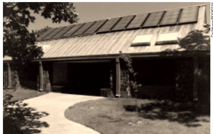
Visitors now enjoy hot showers at Chickasaw National Recreation Area, thanks to solar water heating systems such as the one installed on this large comfort station.
