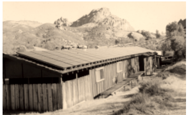
This quiet, unobtrusive hybrid photovoltaic system provides the Chapparral area on the west side of Pinnacles National Monument with clean, reliable electricity. In this pristine area, the photovoltaic installation eliminates park service staff concerns about fuel spills or leaks, because the PV system requires no fuel and produces no emissions.
