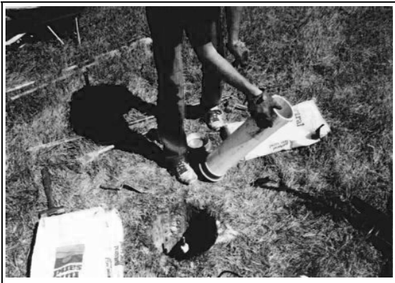
Figure 8.25. Preparing to place 5 or 6 inch PVC pipe over and above the centered grease sleeve and stainless steel rod
