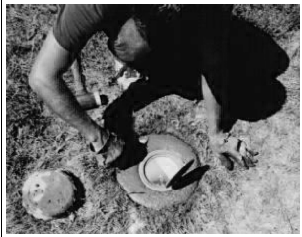
Figure 8.27a. Trowel the top of the concrete until there is a smooth finished surface.
