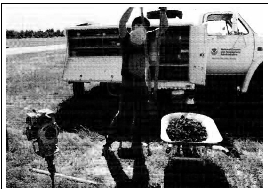
Figure 8.18. Digging the 43" deep hole; 12"- 14" diameter for the top 22" in depth, and 3"- 6" diameter for the bottom 21" (Note, Dirt removed with a wheelbarrow)
