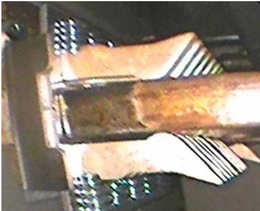
Circuit Breaker Finger & Stab
