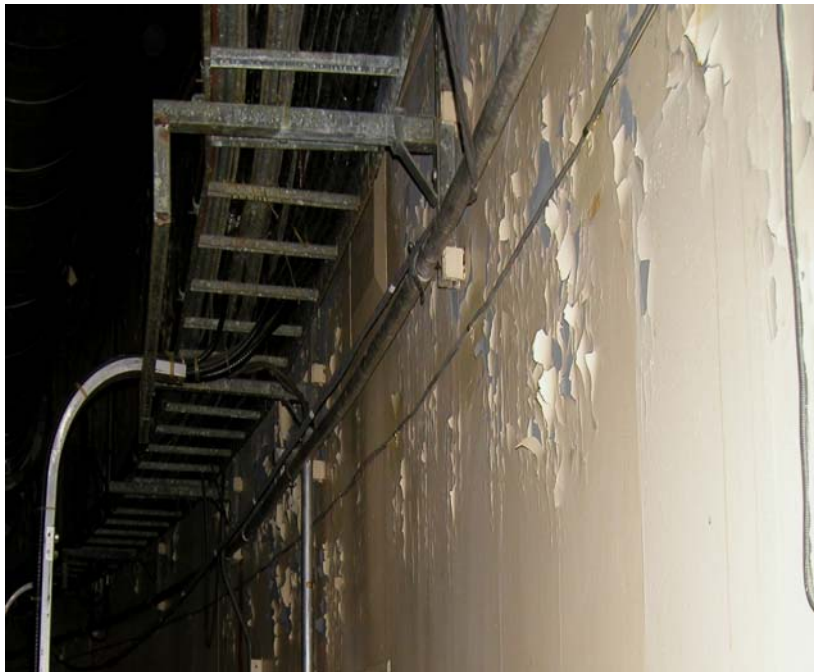
Figure 4 Example of Coatings Degradation at Oconee
