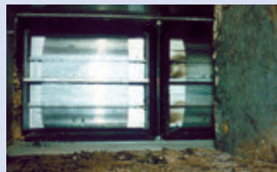
Photo 4C: Moldy air duct
