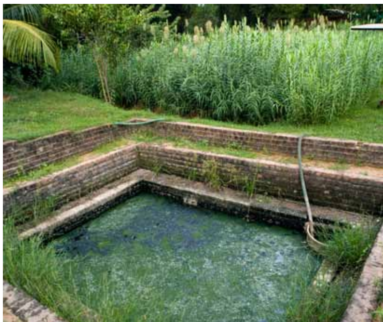
Decentralized wastewater treatment system in Nadu, India, for small volume usage. © Chinch Gryniowicz/SpecialistStock
