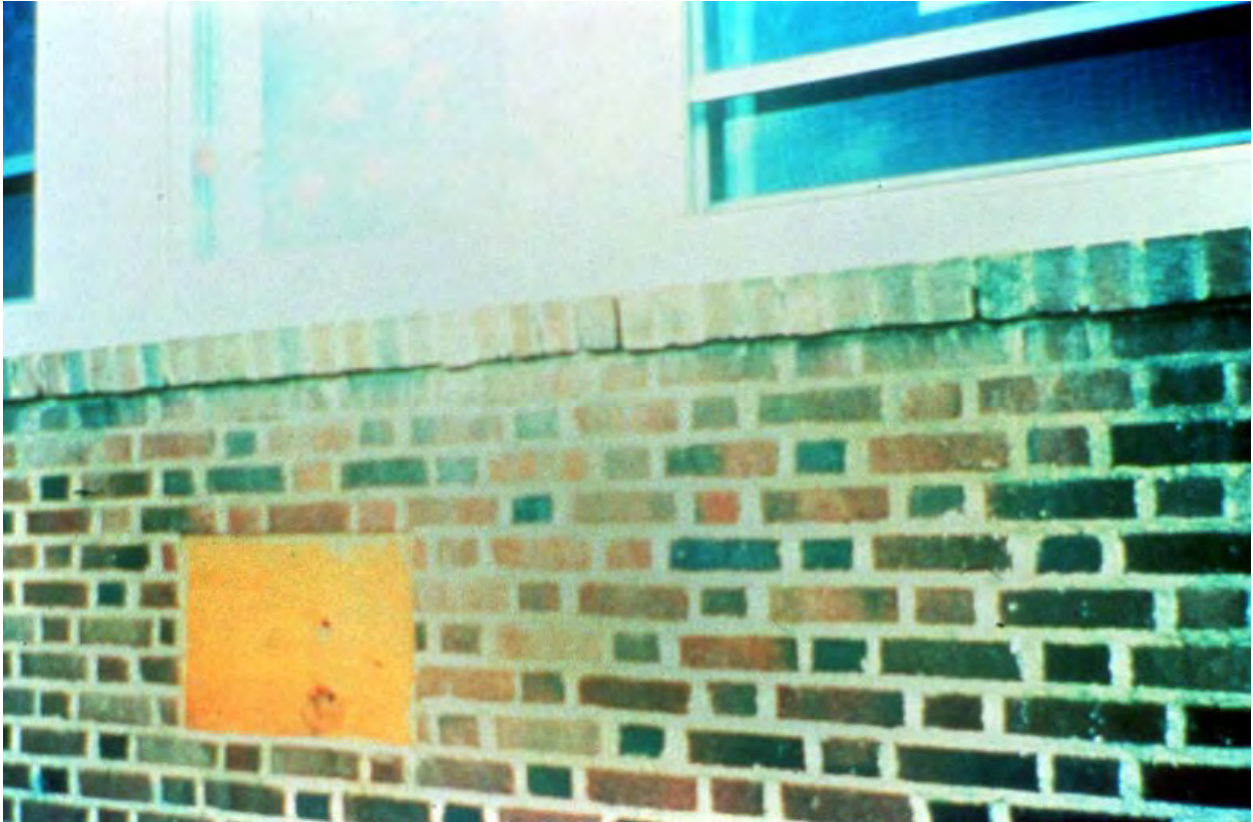
Figure 11 Plywood covering the outdoor air intake for a classroom. Applied during the oil embargoes of the 1970s, the classroom remained under-ventilated until the mid 1980s.
