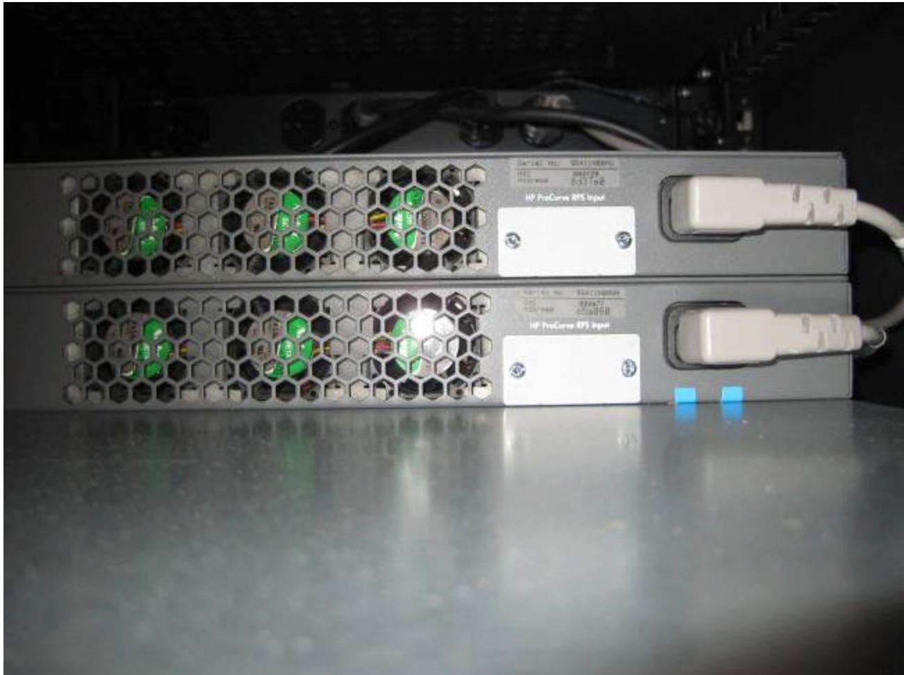
Figure B-2: Hub6/GSW2 Positioned on Top of CHPS4
