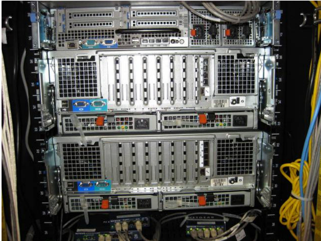
Figure C-2: Rear of REP Rack after Installation
