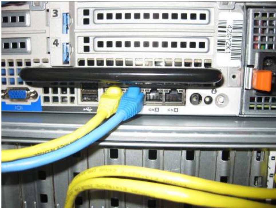
Figure A-8: Dell R710 Ethernet Cable Connections
