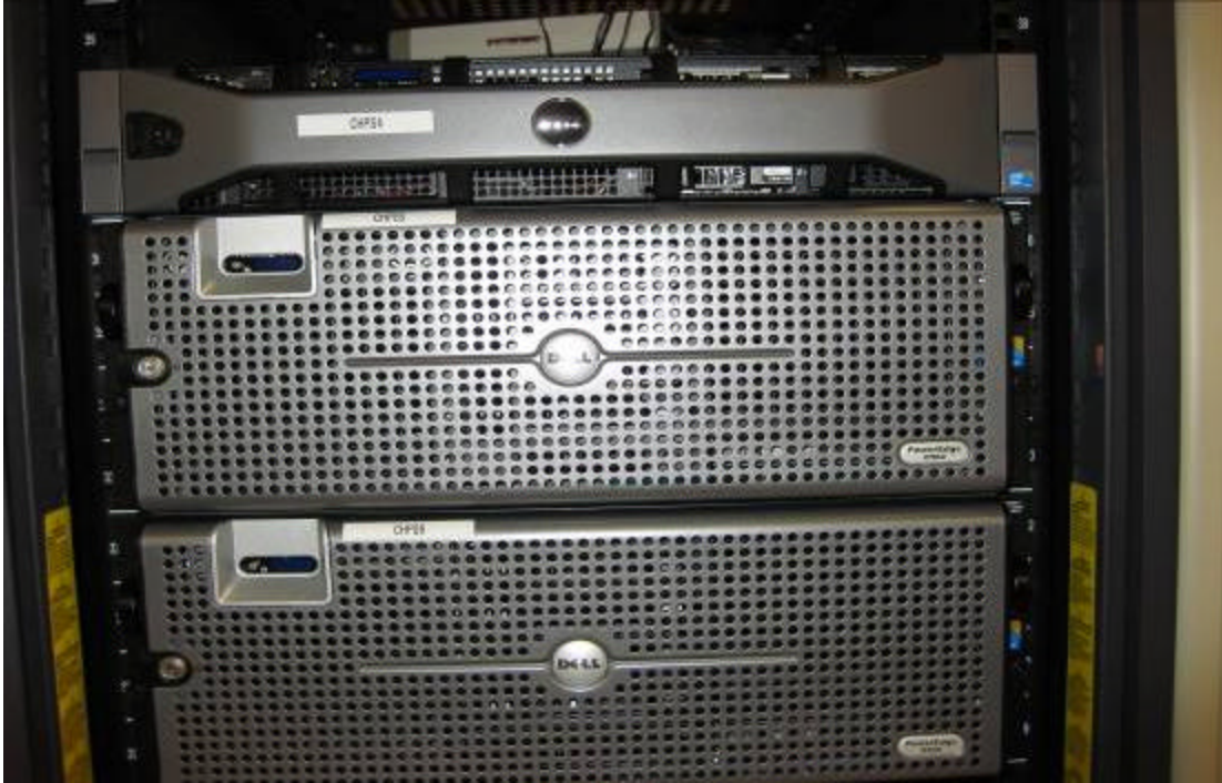
Figure C-4: Front of REP Rack after Installation with Face Covers
