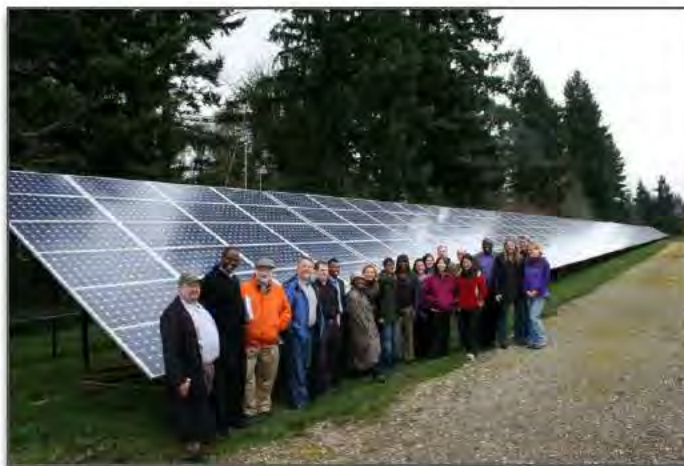
Peer exchange participants at the ODOT Solar Highway Demonstration Project at the Interstate 5 and Interstate 205 interchange in Tualatin, OR. Source: Lynn Frank
