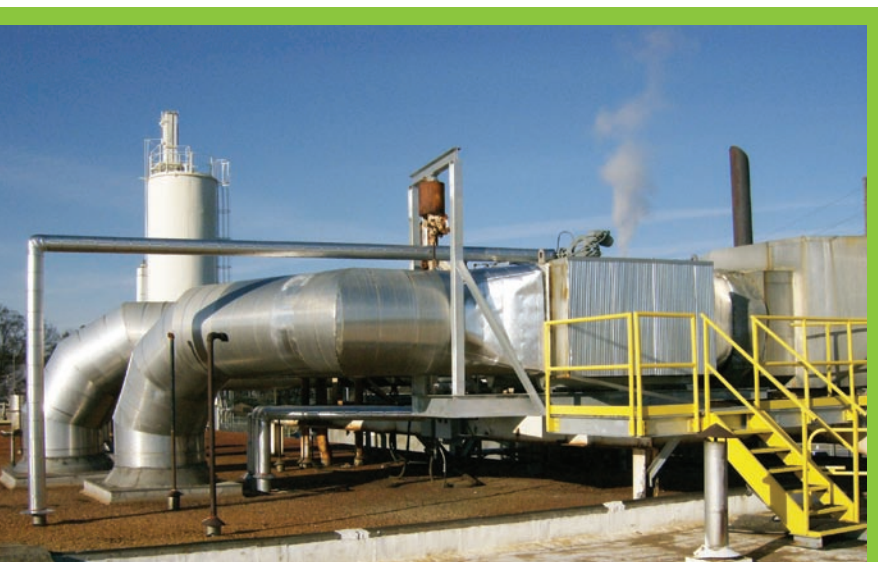
Shaw Industries installed a stack economizer on boiler #3, pictured above, to enable the plant to use excess heat to heat the boiler's feed water.
