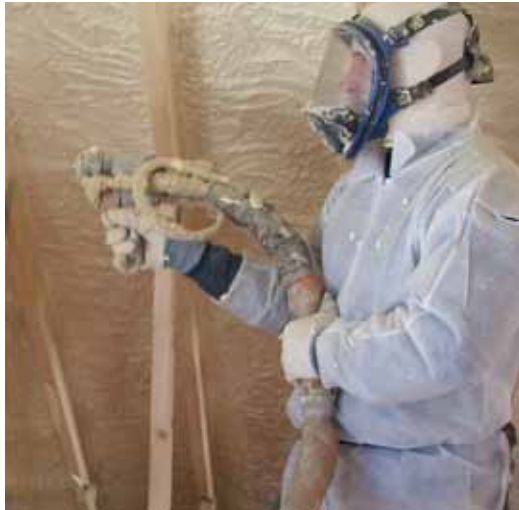
Expensive but comprehensive. Spray foam is applied as a liquid, but quickly foams and expands to fill the insulating space. Photo courtesy of Spray Tech Foam
