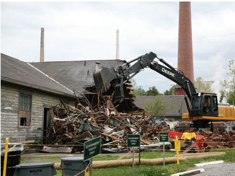
Building 3550, one the last Manhattan Project-era frame structures, was torn down this summer.
