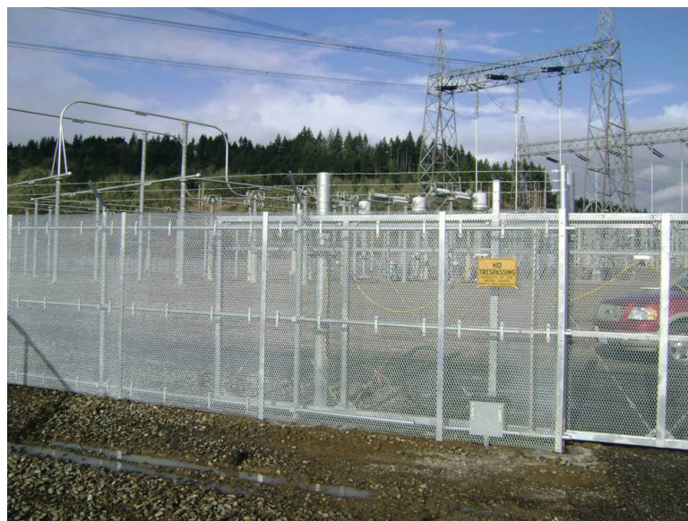
ORNL experts helped install a cost-effective security system to guard a utility substation against copper thefts.
