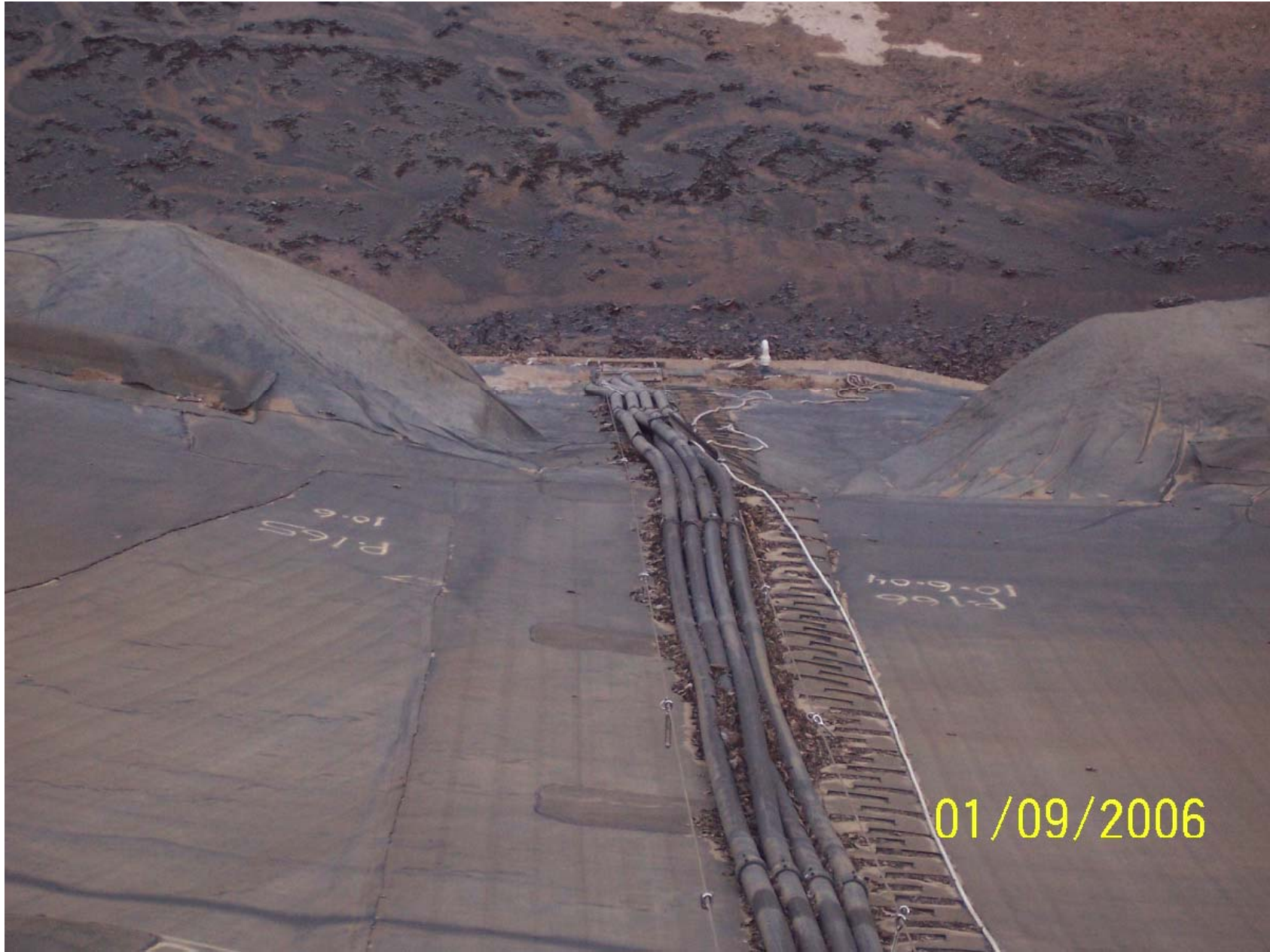
Note separation of guy cable eye bolts from base plates and movement of one pipe over another.
