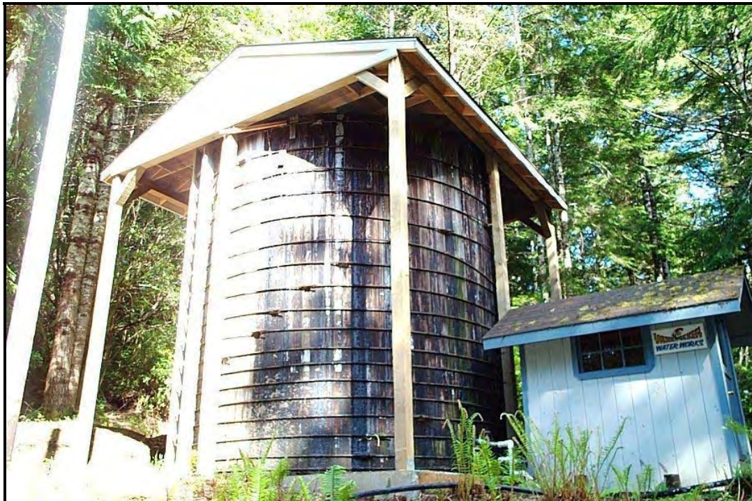
Water tower and structure housing water purification equipment, which serves all buildings on Camp Easter Seal.
