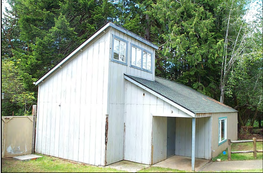
A cottage that has been stripped down to framing on the inside.
