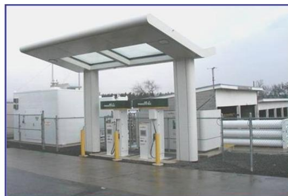
Figure 3.1.1 Distributed hydrogen production facility
