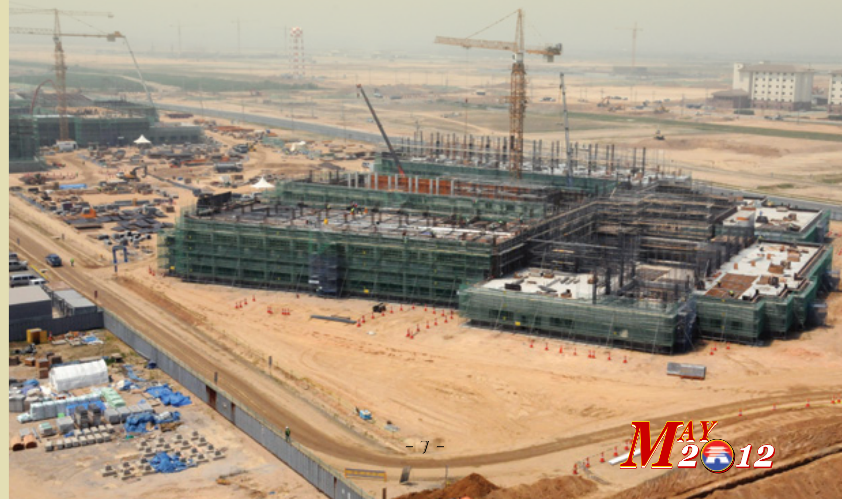
A new elementary school currently under construction at U.S. Army Garrison Humphreys May 25. (Photo by Patrick Bray)
