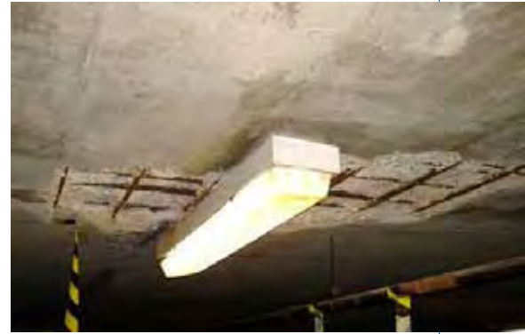
Spalling Garage Roof
