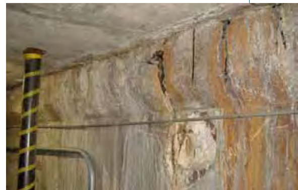
Deteriorated Garage Concrete
