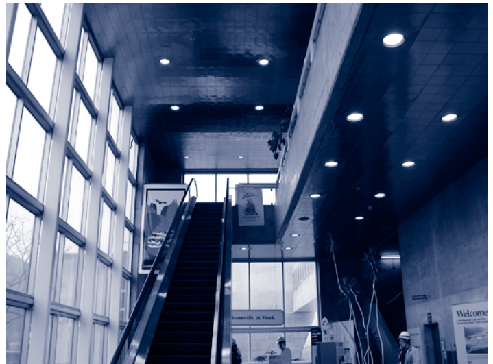
Mercury vapor lighting was replaced with induction lighting in Bonneville Dam's Visitor Center Complex lobby.
