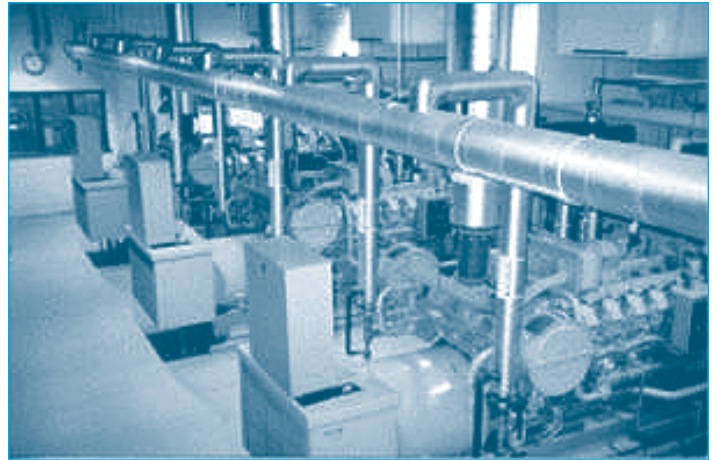
Lean-burn engines designed to generate electricity from landfill gas.
