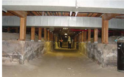
Large crawl space with a walkway. Provides access to plumbing, wiring, and ductwork. PBS does not consider an unfinished crawl space with a dirt floor part of the total constructed area of a building and is not included in the Gross.
