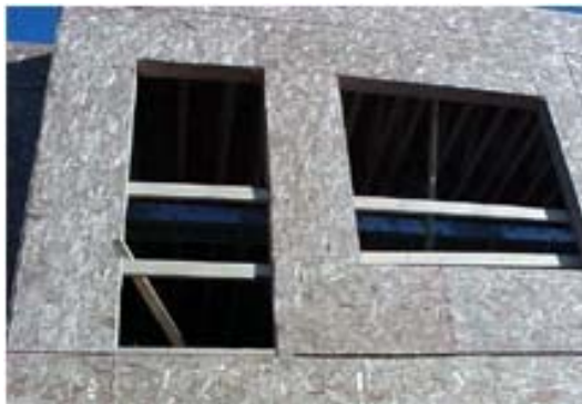
Figure 35 - Guardrails protecting window openings.
