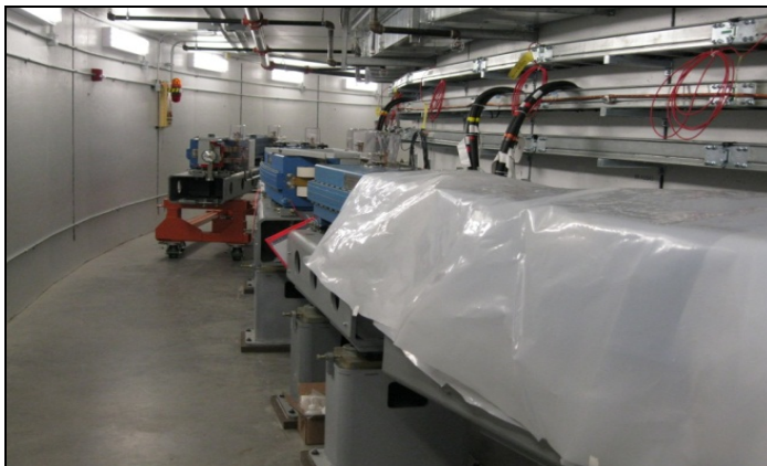
Figure 1. Magnet girders in the booster tunnel.
