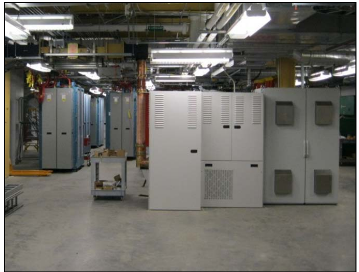
Figure 2. Booster RF transmitter installation.
