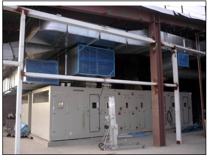
Fig. 6: HVAC equipment in the service building.
