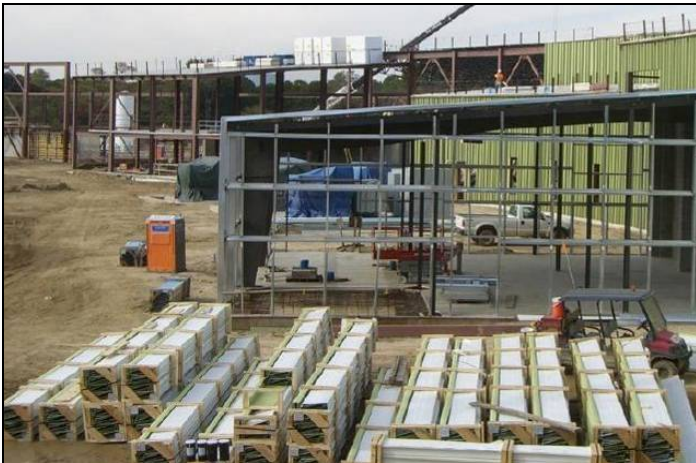
Fig. 5: Compressor building framing, staging for building wall panels, and RF building exterior skin (green) in the background.
