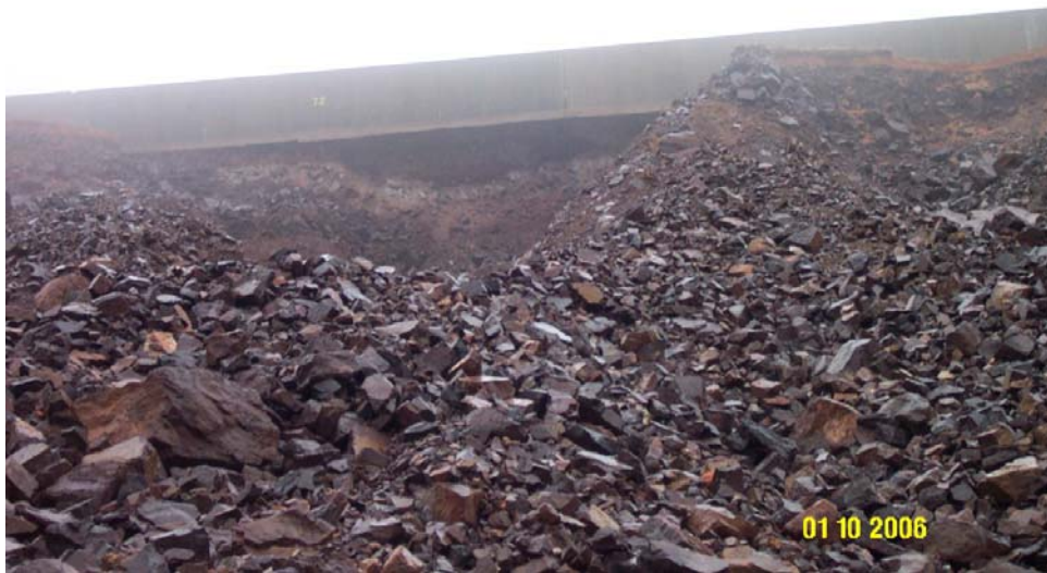
Figure 4.7 - Panel 72 Note erosion deep beneath the parapet wall Damage judged as significant Estimate 0.7 ft of overtopping
