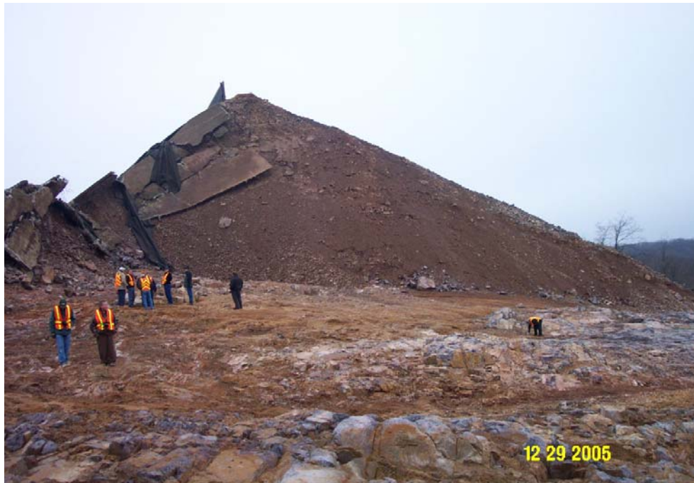
Figure 4.11 - Left side of breach
