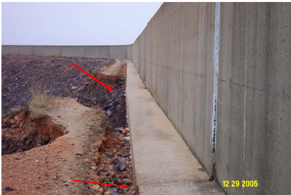
Figure 4.8 - Erosion at Panel 71 footing Note the horizontal displacement between Panel 70 and 71 (foreground) and bowing at the joint between Panels 71 and 72. Erosion at the footing is similar to that described during the September 25, 2005 wave overtopping.
