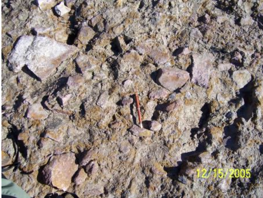
Figure 2.6 - Foundation area composed of weathered rhyolite with some clay, located in breach area.
