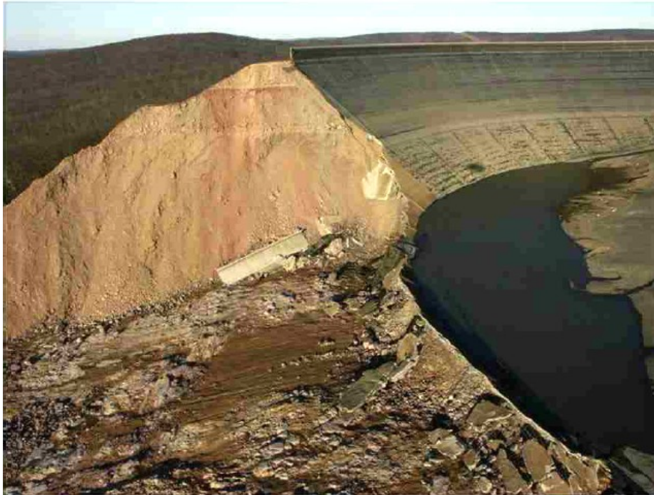
Figure 2.11 - Weathered rock and discontinuous clay seam foundation just downstream of fish-pond area.
