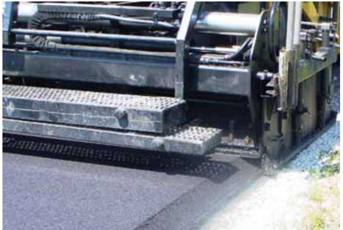
By consolidating the edge of a pavement to 30 degrees, the Safety Edge SM helps mitigate the problem of vertical edge drop-off.
