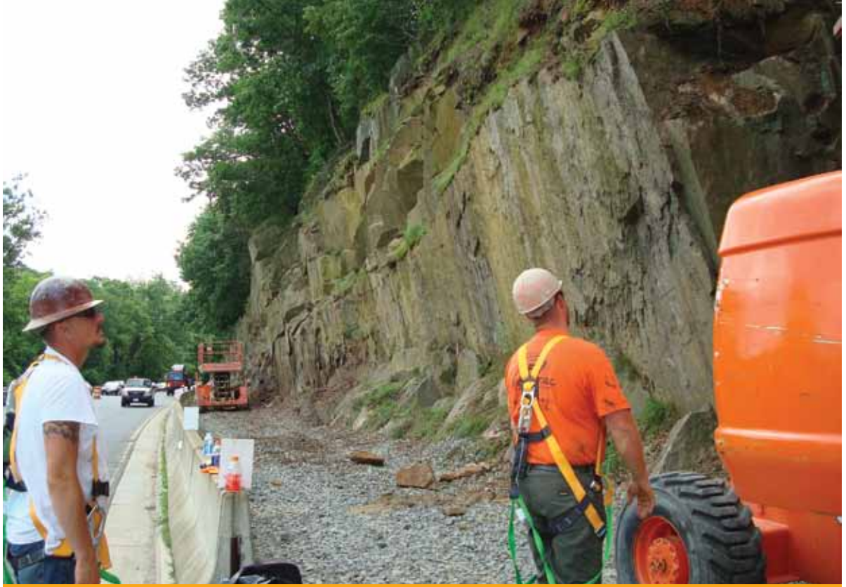
A rock cut slope on the George Washington Memorial Parkway in Arlington, Virginia. The innovative use of rock gluing on the Parkway stabilized the rock slopes while preserving the scenic beauty of the Parkway.
