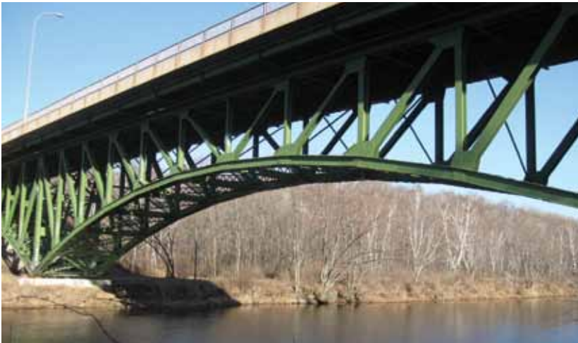
Pilot bridges for the Long-Term Bridge Performance program include this bridge in Sandstone, Minnesota, which carries State Road 123 over the Kettle River.
