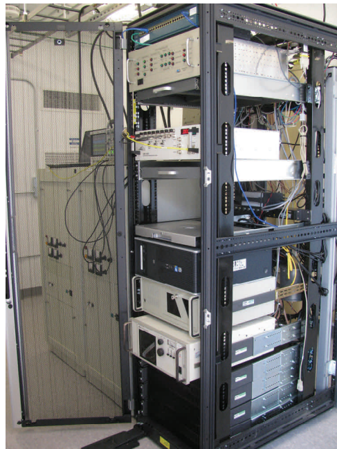
New MRC-520X components at Boise Master Station during field testing. The final system components will have silk-screened front and back panels and be housed in a standard rack mount (July 2012)
