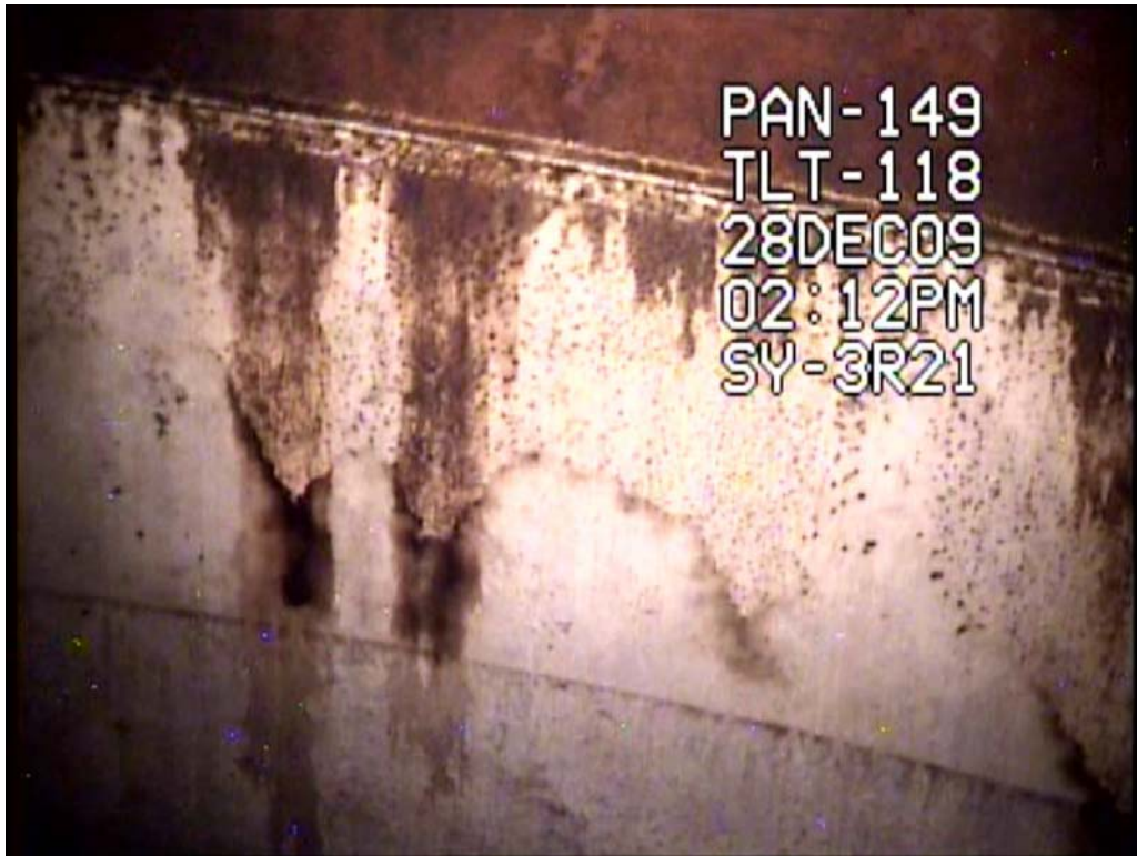
Figure 3-6. Potential Pitting in Tank 241-SY-103 Liquid-Air-Interface Region.
