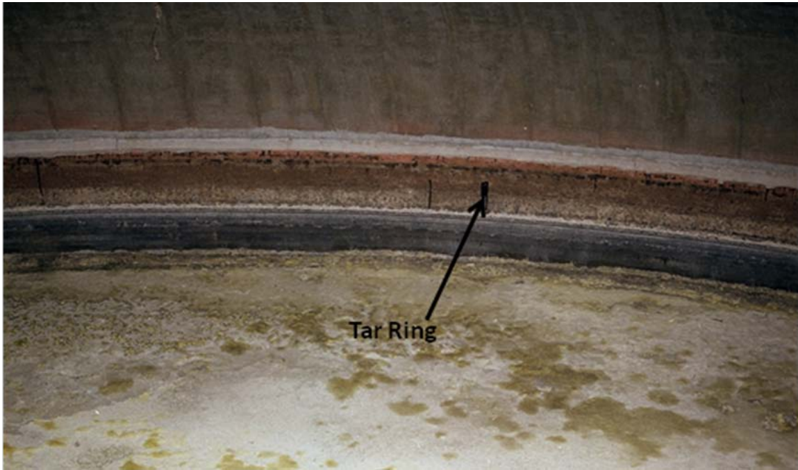
Figure 3-17. Tar Deposits (241-TX-114).
