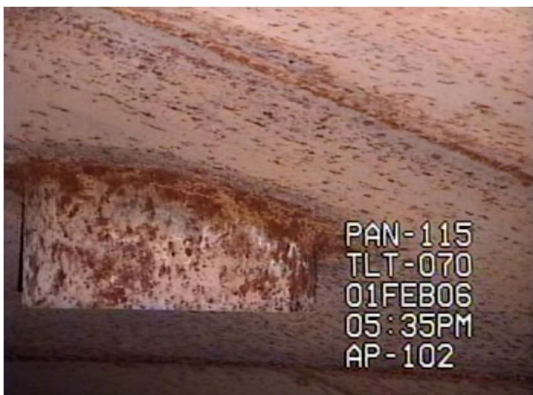
Figure 3-8. Light Corrosion on 241-AP-102 Access Riser Penetration.
