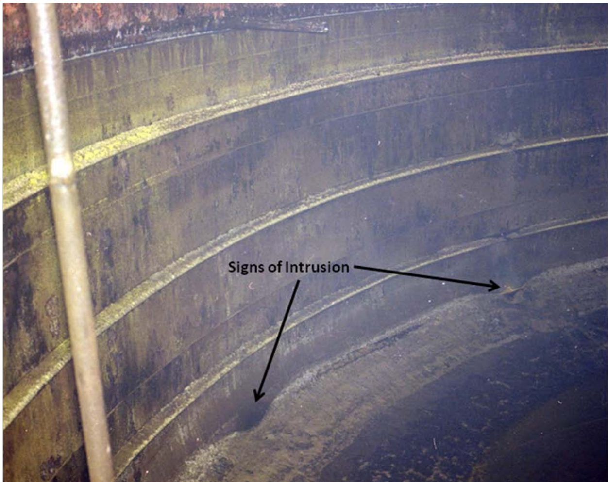
Figure 3-18. Signs of Liquid Intrusion (241-T-102).
