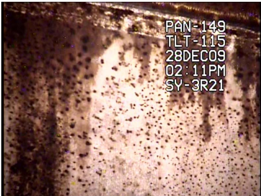
Figure 3-7. Close-Up of Potential Pitting in Tank 241-SY-103 Liquid-Air-Interface Region.
