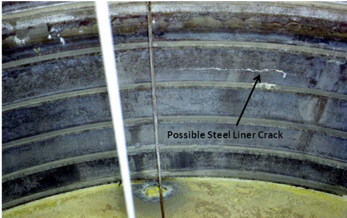
Figure 3-19. Possible Steel Liner Crack (241-SX-112).
